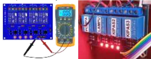
Gambar 33. Kondisi relay high
