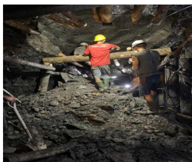
Gambar 2. Ambruk Atap Tunnel THC 04
