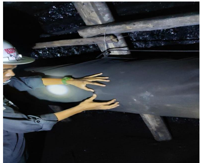
Gambar 1.kebocoran duct di lubang 02 PT. Cahaya Bumi Perdana
