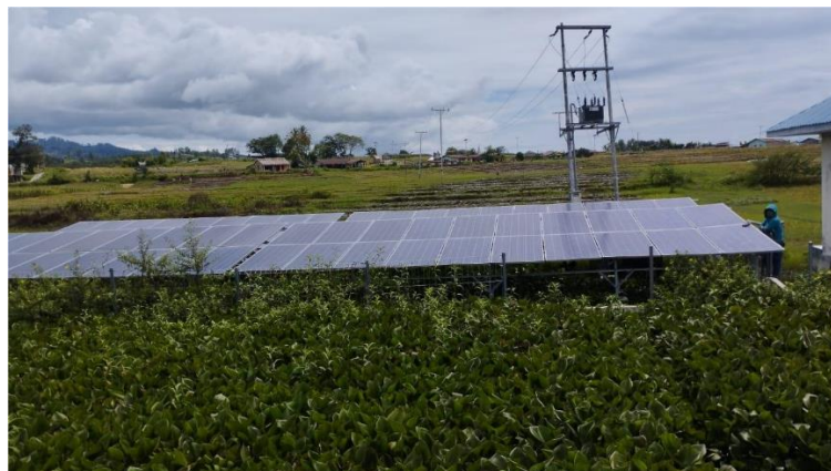
Figure 6. The condition of the PLTS Array at the research location in Palipi
