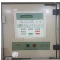
Gambar 3 Remote Terminal Unit/Feeder Terminal Unit
